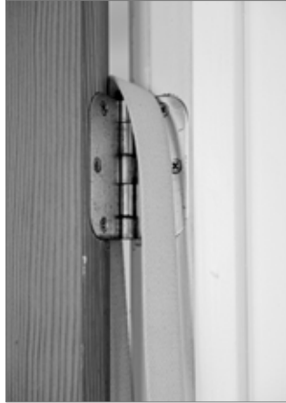
Figure 6.5 Set-up 1 on a door hinge
